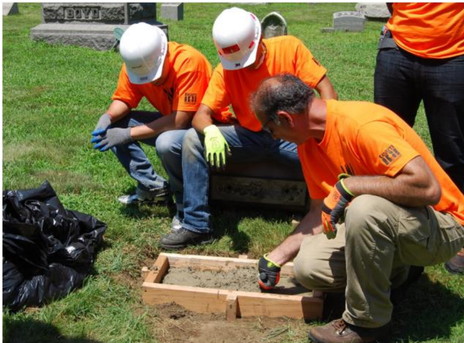
Trainees working with a resident craftsman (Cleaning a roof as part of the Woodlawn Bridges to Crafts Careers Preservation Training Program (Woodlawn Cemetery & Conservancy))
